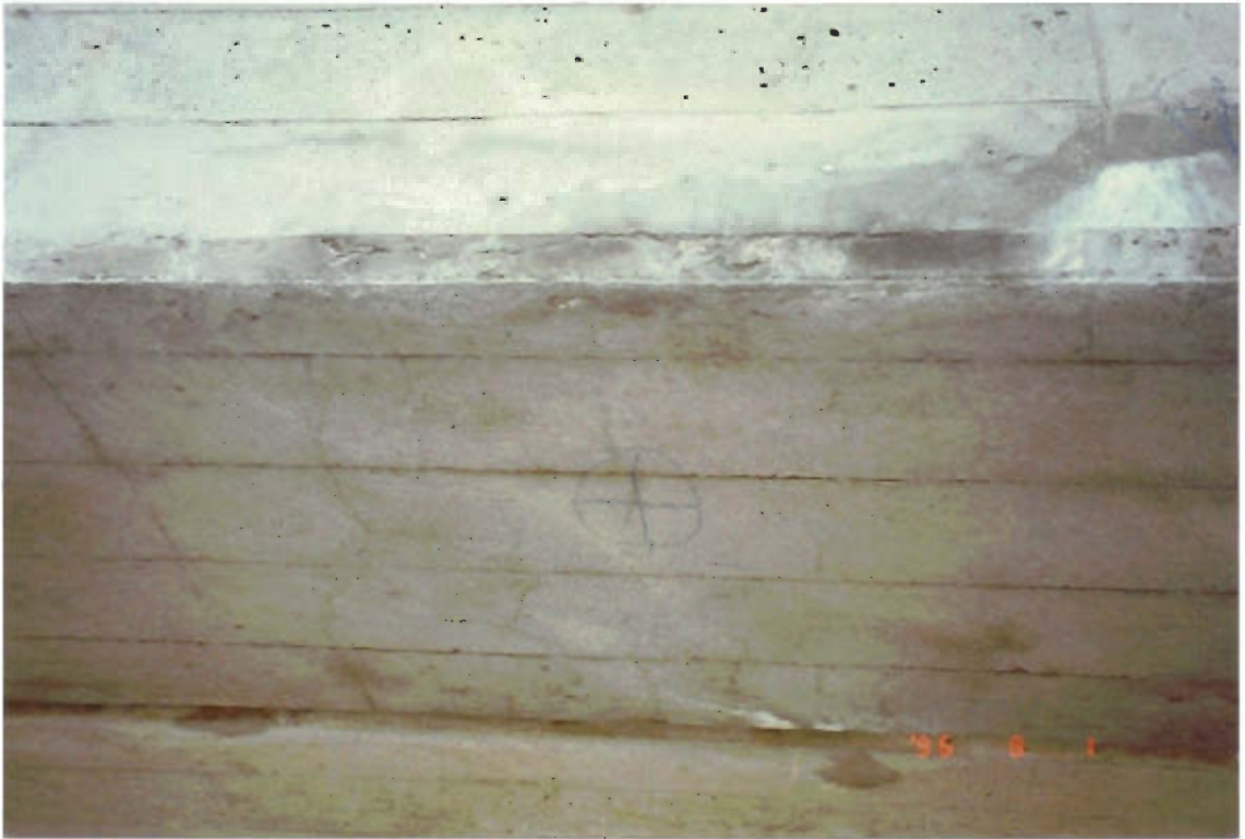
Figure 9: Repair under the edge of the bridge girder of bridge 3 - shotcrete repairs from 1978. Visual observations of the repairs are single cracks and white extrusions on the surfaces.
