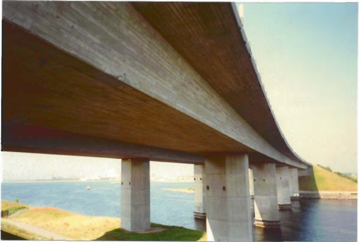
Figure 5: Bridge 3 was built in 1981. The defects which were inspected were holes from bad compaction in the bottom part of the slab due to lack of space between the prestressing ducts. The defects were repaired with shotcrete.
