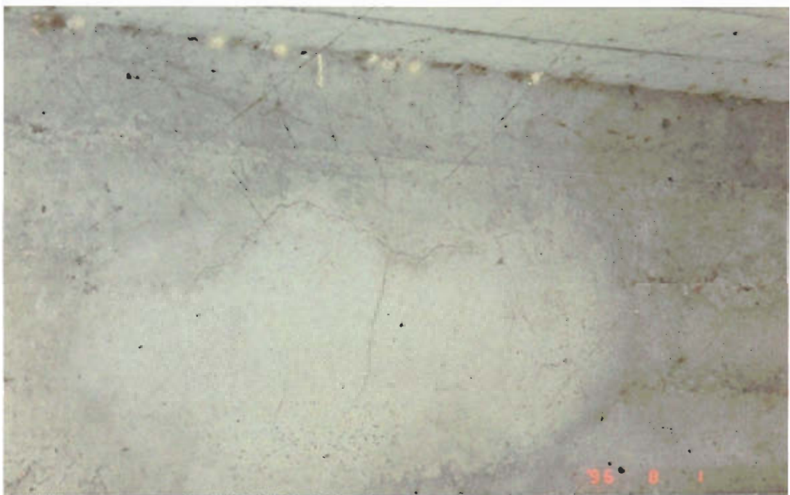
Figure 10: Repair under the middle of the bridge girder of bridge 3 - shotcrete repairs from 1978. Visual observations on the repairs are single cracks.
