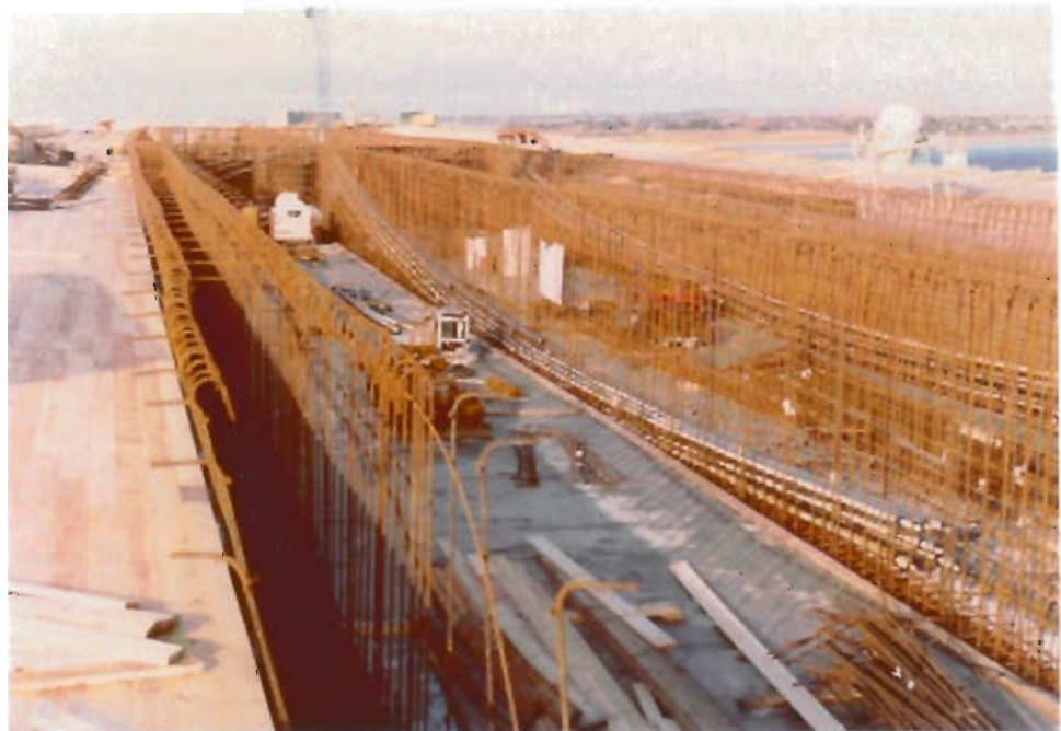
Figure 6: Bridge 3 during the construction phase. Reinforcement and prestressing ducts arranged before casting at the box girder.
