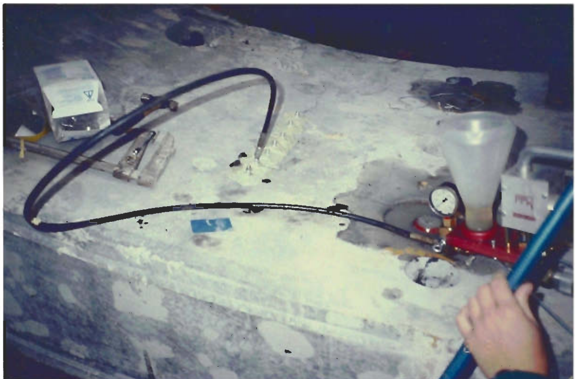
Figure 21: (Photo: E. Kluge) Injection of cracks with epoxy resin. Nipples are glued to the concrete surface on the top of the crack.
