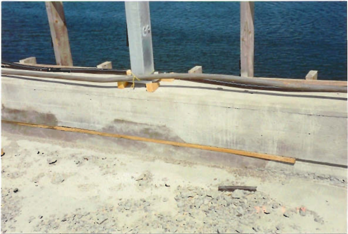
Figure 3: Repairs at the inner corner of the edge beam on bridge 2. The defect was caused by settlement of the concrete at very early age.
