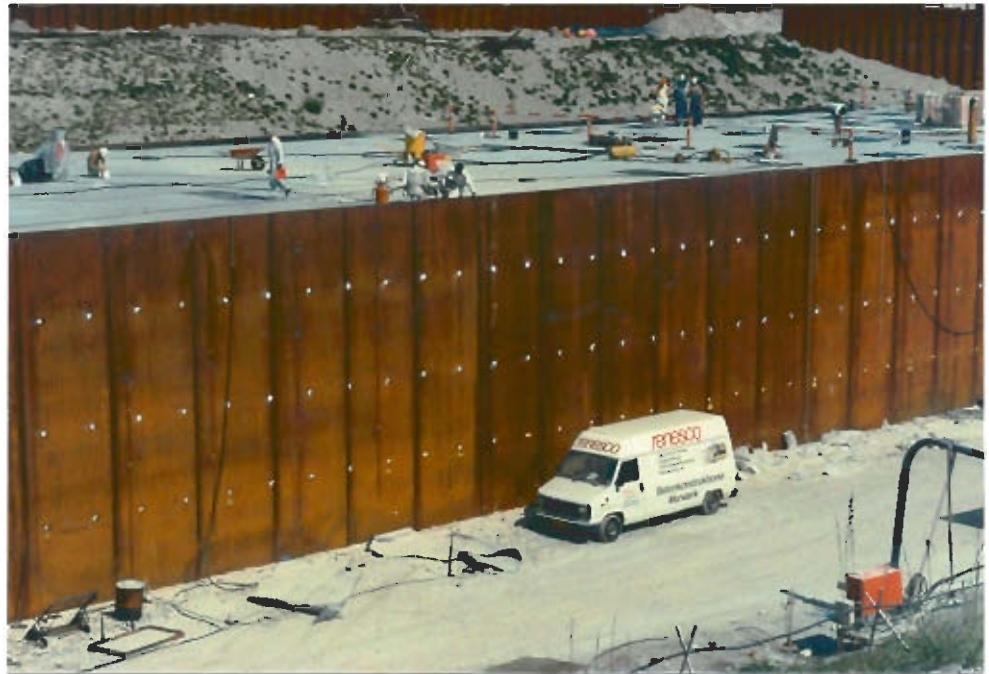
Figure 20: (Photo: RENESCO) Injection of cracks on the top deck of a tunnel. The injection included more than 900 injection valves in drilled holes and more than 900 litres of acrylic injections materials were used.
