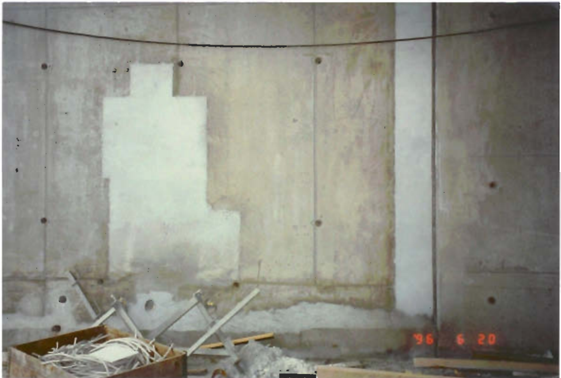
Figure 4: The tunnel was built in 1996. The six repairs which were inspected were located on the inner side of the tunnel walls from 0-2 m above bottom slab level. The defects were holes and porous areas due to bad compaction or due to ice and snow in the bottom part of the form. The holes and porous areas were repaired with repair concrete (similar to the construction concrete), mortar or shotcrete respectively.
