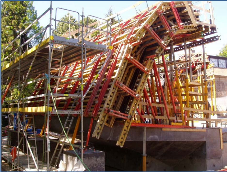
Fig. 4: Complex formwork for the Ordrupgaard extension manufactured with a high level of craftsmanship.
