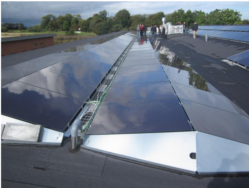
East-West installation with a-Si modules on the roof of Marienlyst old peoples home. Skive 18 September 2012
