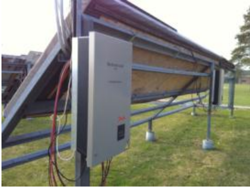
Figure 6.1 Electronic load connected to solar modules
