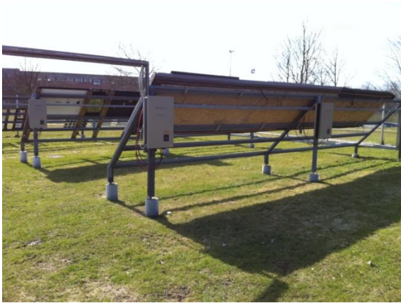
The two module racks seen from behind.
