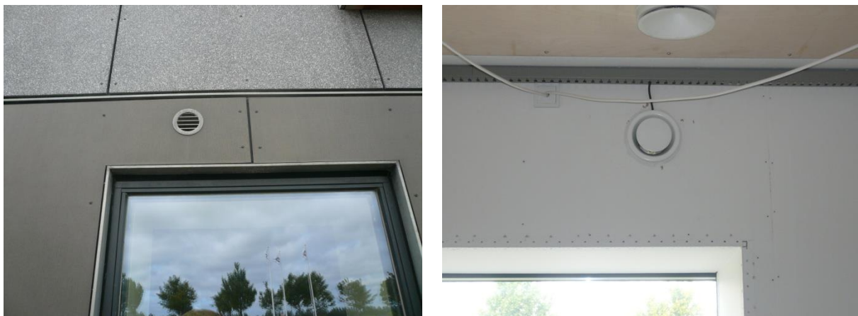
Figure 2.5. One of the operable fresh air valves seen from the outside and the inside.
