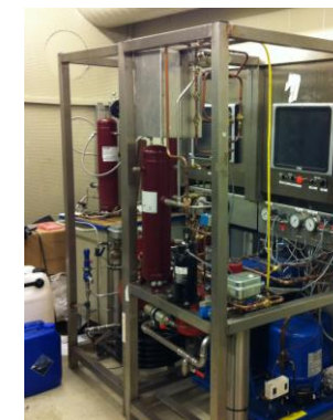
Test of heat pumps.
