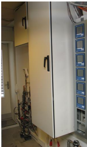
Heat meters at EnergyFlexLab.
