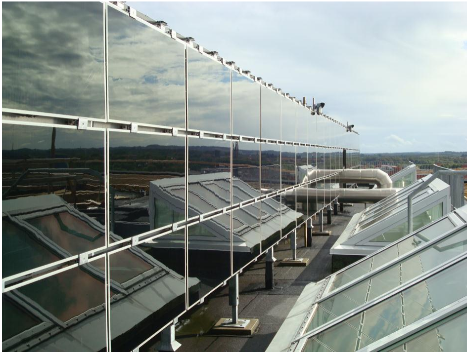
Skive Townhall, CdTe-modules. 18 September 2012
