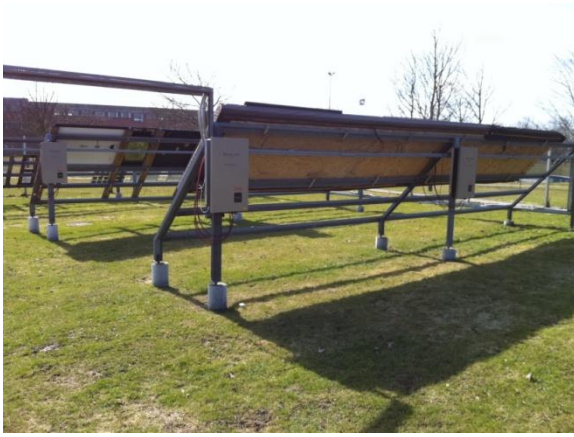
The two module racks seen from behind.
