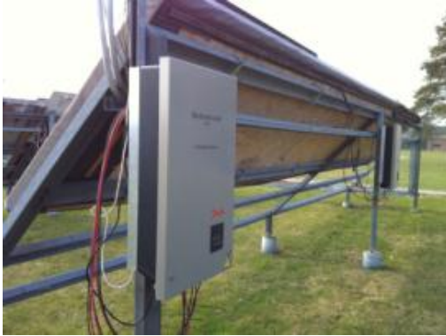
Figure 6.1 Electronic load connected to solar modules
