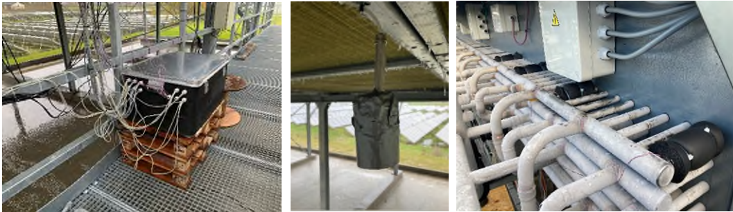
Figure 135: Measuring box, air temperature sensor and temperature sensors on pipes.
