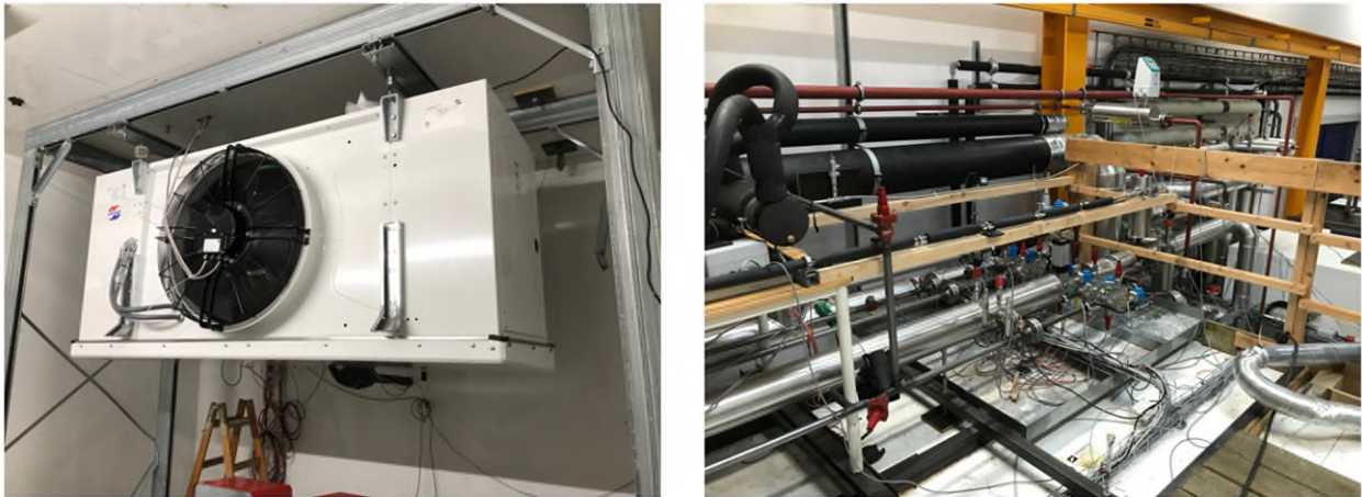
Figure 80: Evaporator to the left and valve station to the right.
