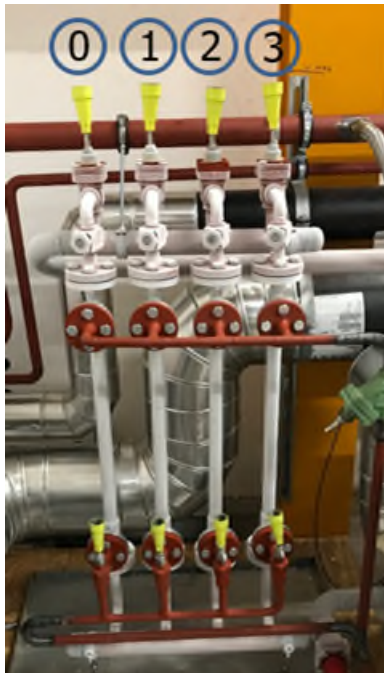
Figure 90: Suction gas heat exchanger SGHX.
