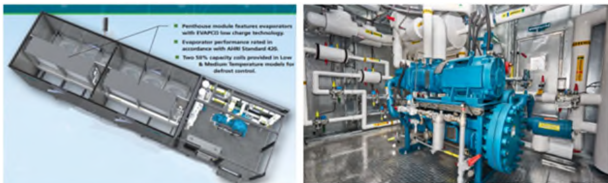
Figure 17: Unit from Evapcold on the left, and machine room on the right.
