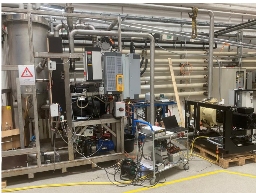
Figure 32: Installation of the uHeater at the test rig at Danish Technological Institute.
