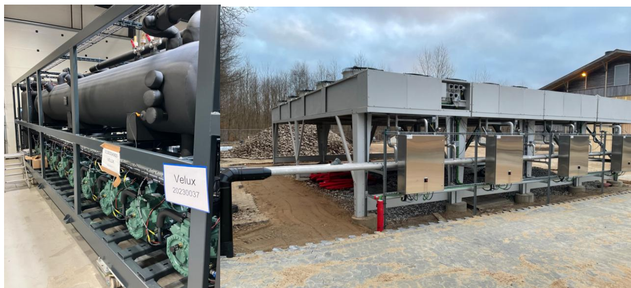
Figure 5: The heat pump and air source heat exchangers at the field test site.
